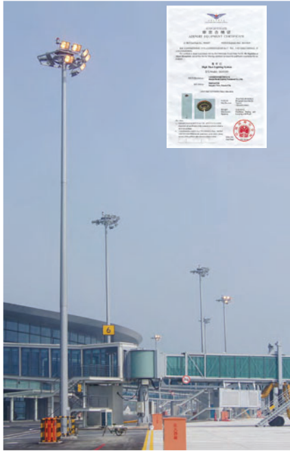
扬州泰州机场高杆灯 YANGZHOU TAIZHOU AIRPORT HIGH MAST LIGHTING PROJECT
